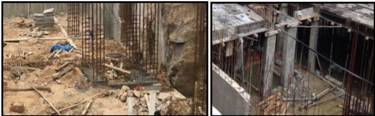
Figure 3.1 & 3.2: Debris lying around on site
