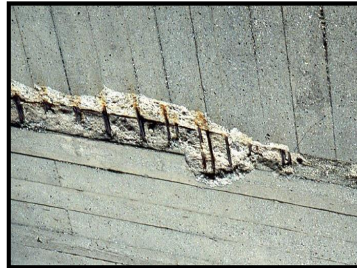
Figure 2.3: Concrete cancer (Cracks)
